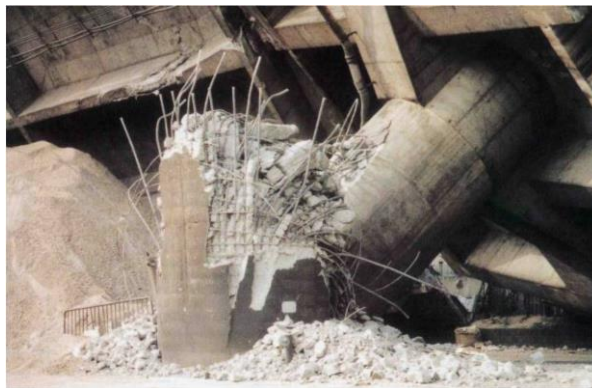
Figure 1.12 Failure of column with terminated longitudinal reinforcement in the 1995 Hyogo-Ken Nanbu Earthquake
