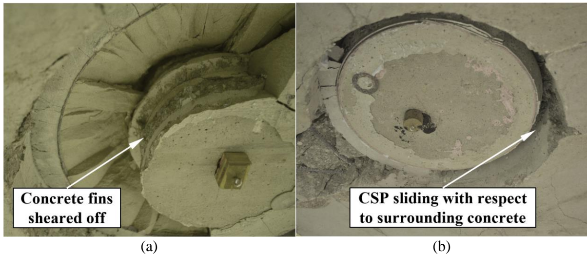
Figure 3.4 Failure modes: (a) column segment-to-grout interface failure; (b) CSP-to-foundation interface failure
