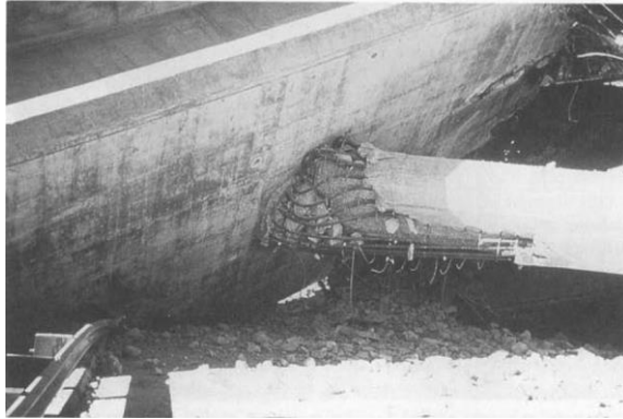
Figure 1.10 Confinement failure of column in the 1971 San Fernando Earthquake
