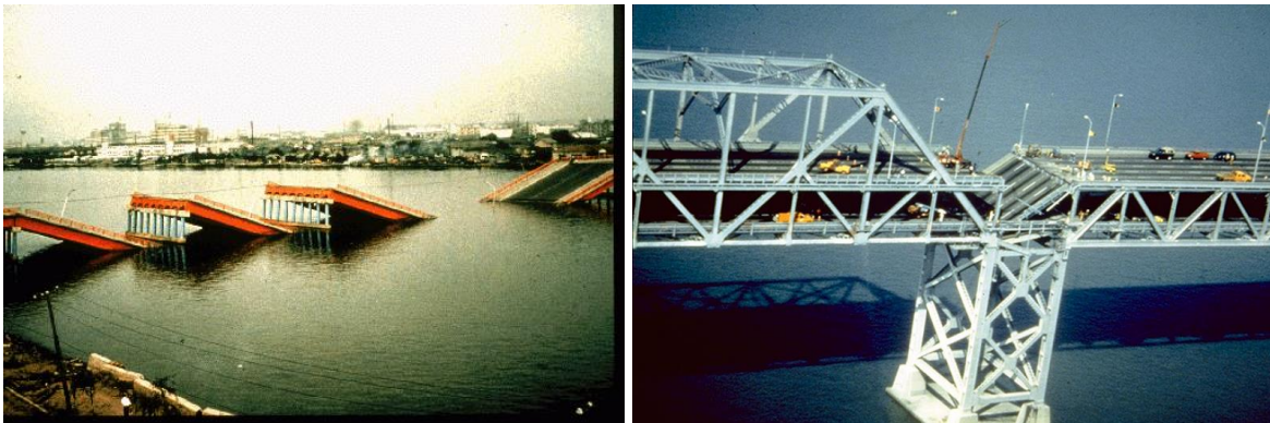
Figure 1.9 Span unseating in the 1964 Niigata Earthquake (left) and the 1989 Loma Prieta Earthquake (right)
