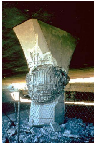
Figure 1.11 Shear failure of a column in the 1994 Northridge Earthquake
