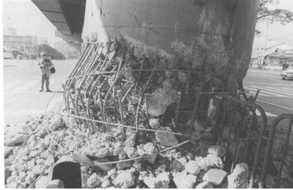
Figure 1.13 Weld splice failure of column longitudinal reinforcement in the 1995 Kobe Earthquake
